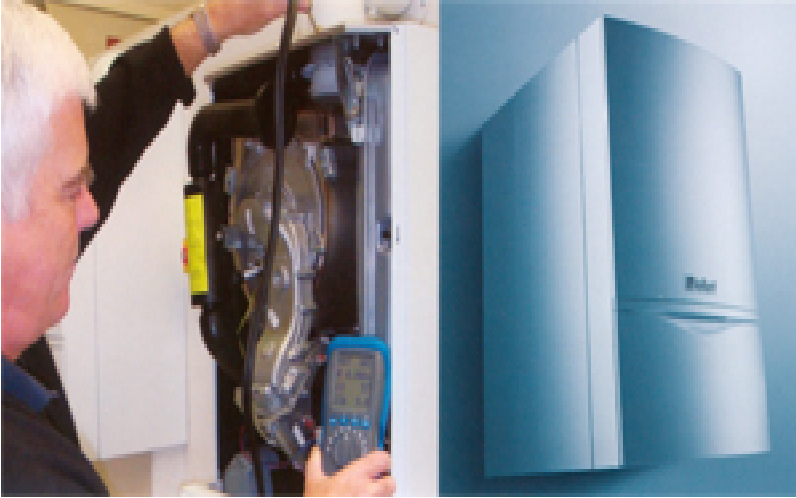
Combustion Performance Assessment
